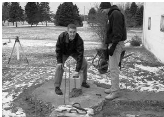
Pastor Doug McMunn lays cinderblock for Arise Church foundation, as Mark Donovan looks on.
